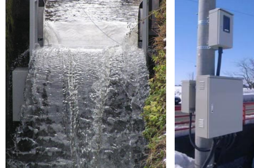
Fig.3 Micro hydraulic turbine installed at drop & power system interconnection equipment
